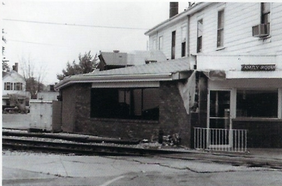
New Albany offered a couple of very tight situations. Above, a portion of roof had to be removed from Tommy Lancaster's restaurant to permit the load to pass. Below, workers keep a close eye on another tight squeeze.
